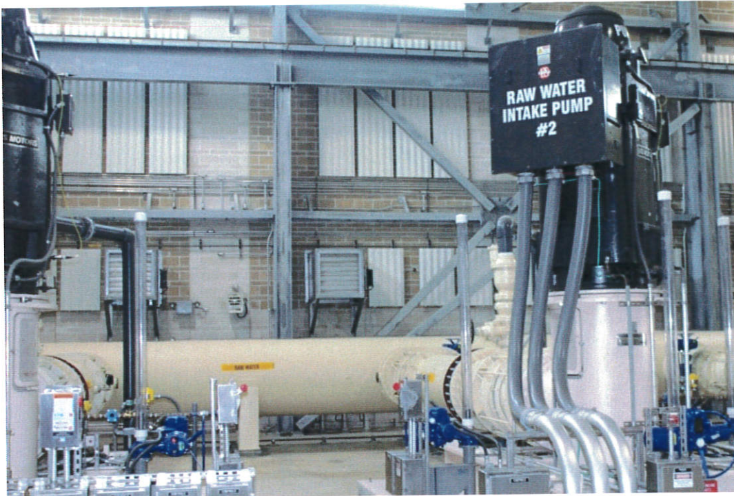
The San Jacinto River Authority's surface water treatment plant was built as part of its groundwater reduction plan, an effort to make Montgomery County use more surface water. (Community Impact staff)
